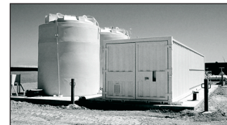
City of Avondale 2000 GPM Nitrate Removal
