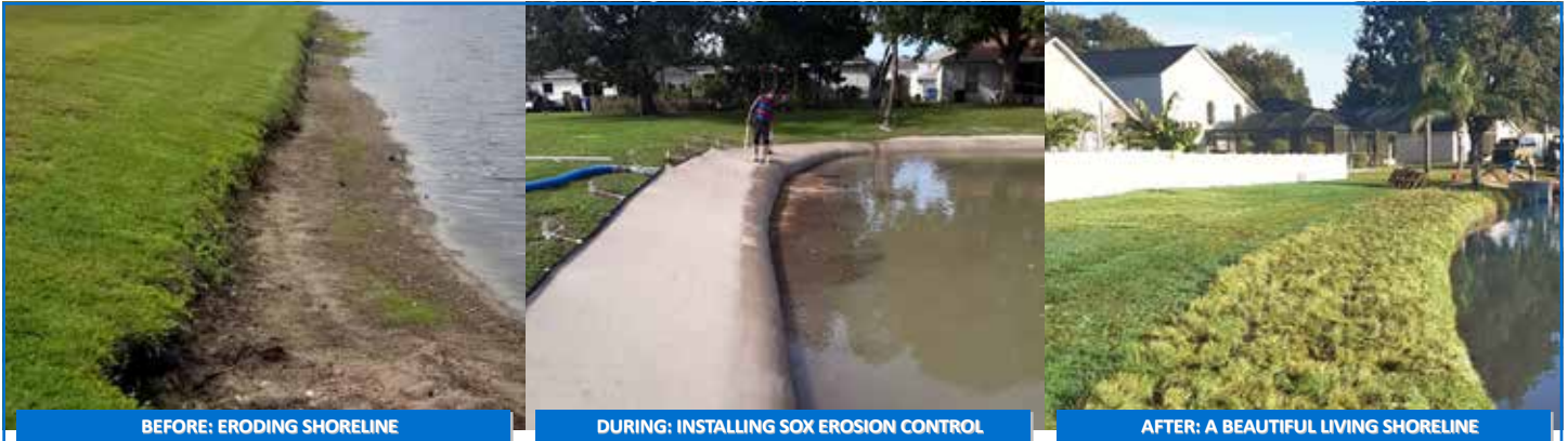
BEFORE: ERODING SHORELINE
