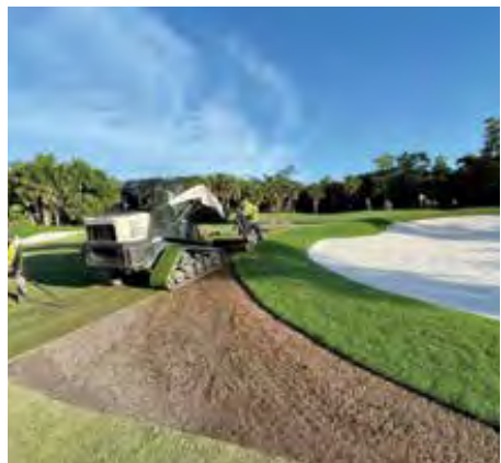
Top: As part of the renovation, all of the sand was removed from the bunkers. The Better Billy Bunker method was utilized in the reconstruction and new bunker sand was added.
