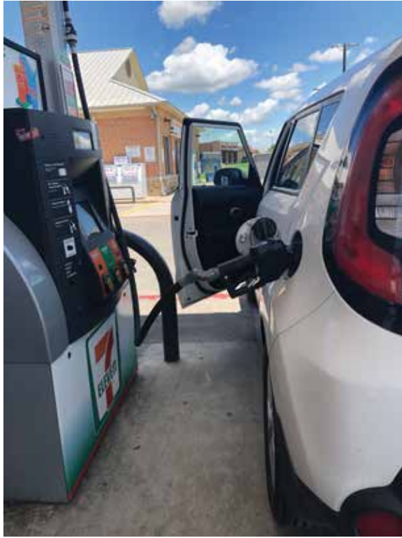
Photo 1.02 Typical motor fuel dispensing facilities fall under the requirements of Article 514 of the NEC ; NFPA 30A is the associated standard.
