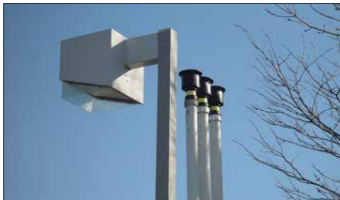
Photo 1.01 Class I, Divisions 1 and 2 areas within determined distances from underground gasoline tank vents
