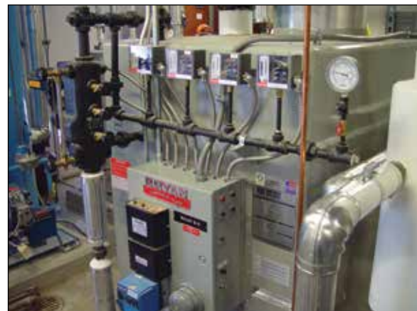
Photo 1.03 A natural gas boiler with a sealed gas piping system
