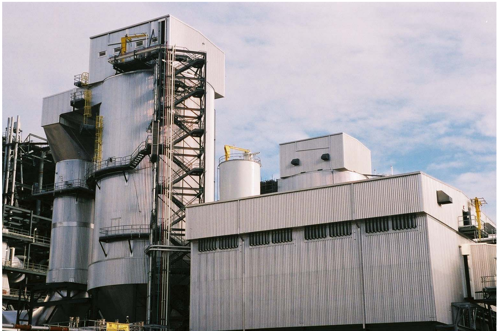
Figure 3. JEA Northside Unit 2, WAPC Spray Dryer Absorber/Fabric Filter
