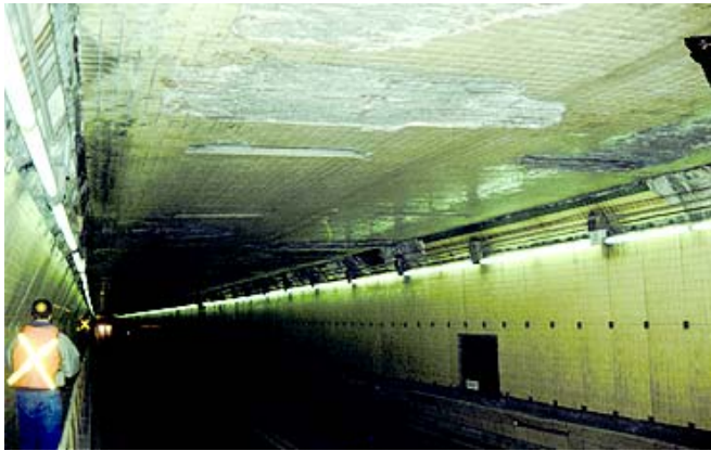
Figure 1: Tunnel prior to repair
