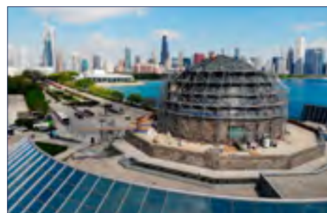
(From top down) The Adler's original roof under construction, fall of 1929. Adler's first roof replacement, June 13th, 1940. The condition of the domed roof before the second replacement began, April 10th, 2021. Scaffolding going up around the dome, April 21st, 2021. The slightly different than normal view of the Chicago skyline, May 6th, 2021. All courtesy of Adler Planetarium.
