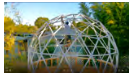
(From top). The floor platform is complete.; The first section of the dome structure is up; The geodesic structure is complete! Images: All photos courtesy of James Hicks
