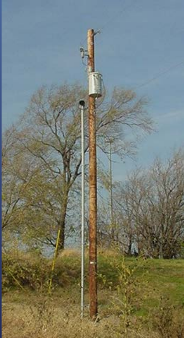
← Single Phase 25KVA Xfmr
