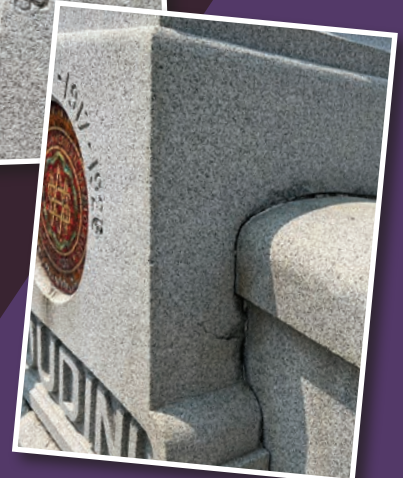
Large cracks in the stone monument have been increasing in size due to age and weather.
