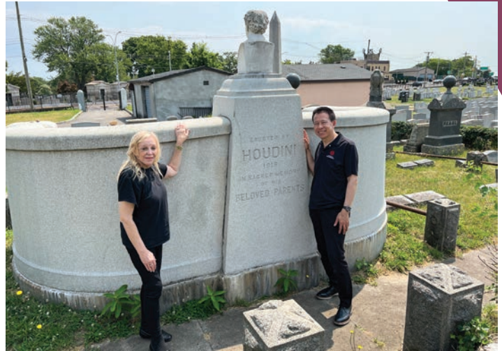
Dorothy and Rod at the back of the gravesite. Note the large cracks along the upper left side.
