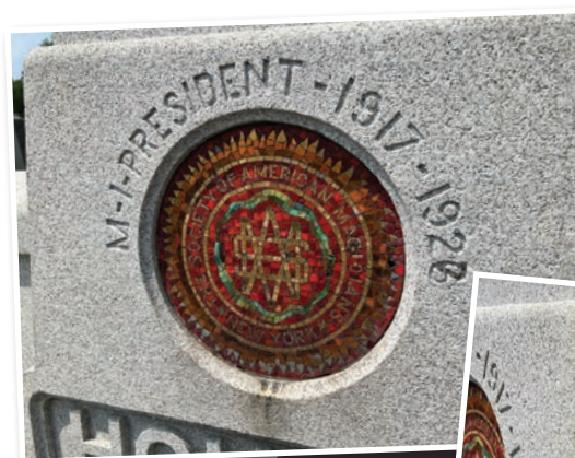
The stonework and the colorful seal are all in need of repair.
