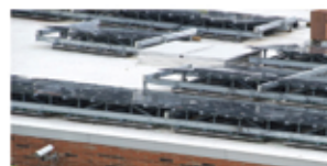
Photovoltaic Roofing System on White Reflective Roof
