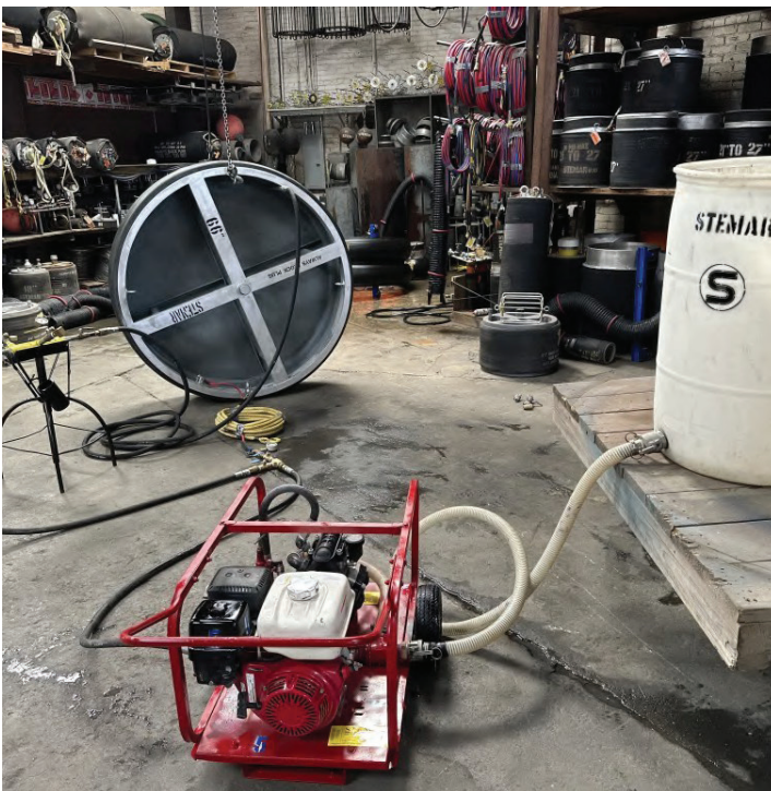
66" high-pressure test plug set up for inflation and test through via hydro-pump
