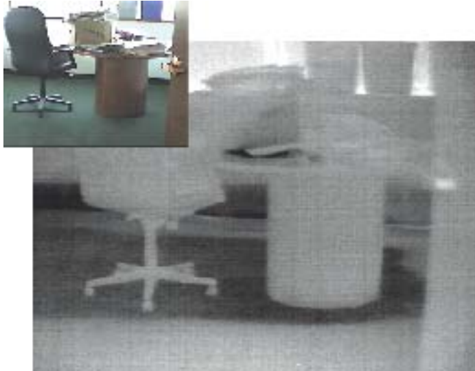
Figure 4. Chair and Carpet. The thermal pattern clearly indicates that moisture remains in part of the carpet and in the lower portion of the wall
