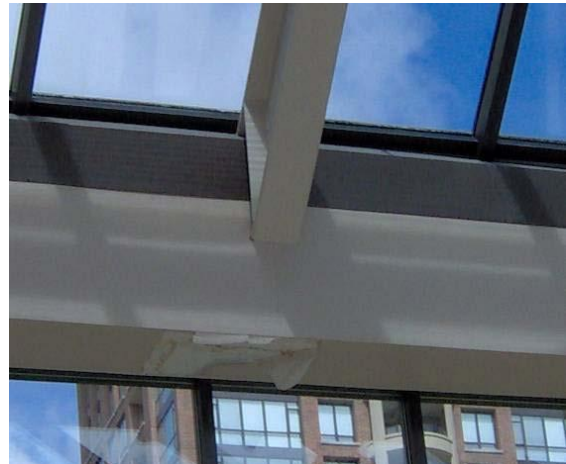
PHOTOGRAPH 13: Damage to the ceiling caused by the leaking of a very large skylight without the raised leg overlapped drainage gutters.
