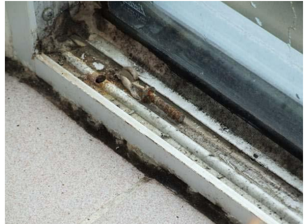
PHOTOGRAPH 11: The window shown on Figure 2 was utilized on a building and leaked. The windows were converted to a rainscreen water management approach by drilling weep holes through the extrusion and installing a fillet bead of sealant (heel bead) at the location marked by the red arrow.
