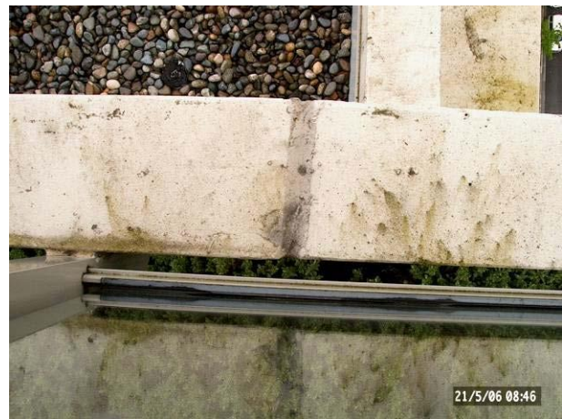
PHOTOGRAPH 7: The top of this parapet wall, on a building located approximately 10 blocks away from the building shown on Photograph 5. In this case, a joint in the parapet wall is waterproofed with sealant, thus increasing the likelihood of leakage.
