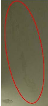
PHOTOGRAPH 4: The ellipse denotes a crack in the ceiling where water was dripping.
