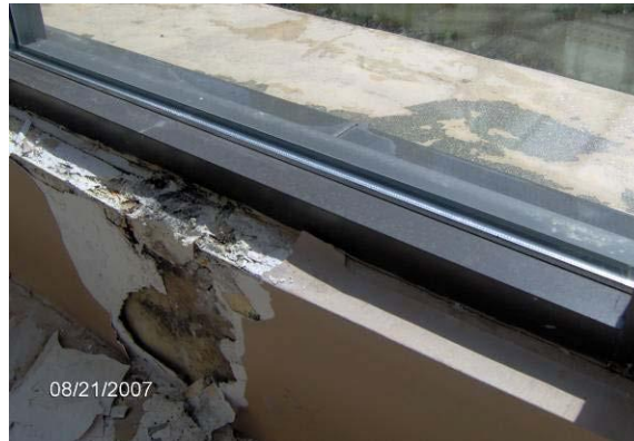
PHOTOGRAPH 10: Shows the consequence of utilizing a storefront window system in a location exposed to wind-driven rain without adequate sub-sill waterproofing. The sub-sill flashing in this photograph had a joint at the point of the leak.
