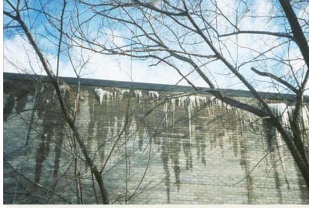
Figure 1: Example of a disconnect between wall and roof air barriers
