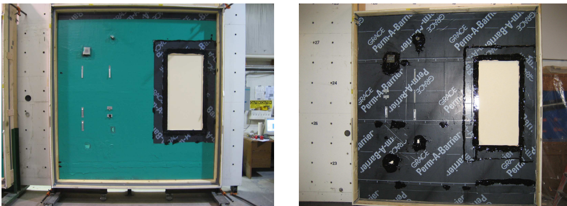
Figure 9: Full scale mock-ups of the installed air barrier assemblies complete with PVC pipe HVAC duct and electrical box penetrations sealed, windows flashed, tie-ins to roof and foundation and post-applied brick ties.
