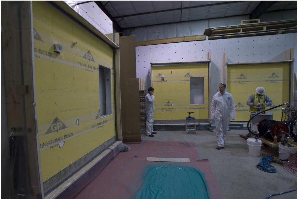
Figure 5: Photograph of wall specimens tested by Intertek. Each wall specimen was constructed according to ASTM E 2357 specifications.
