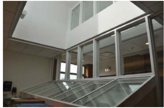
Figure 18: Upper level south facing classroom light well and clerestory monitor ceiling opening
