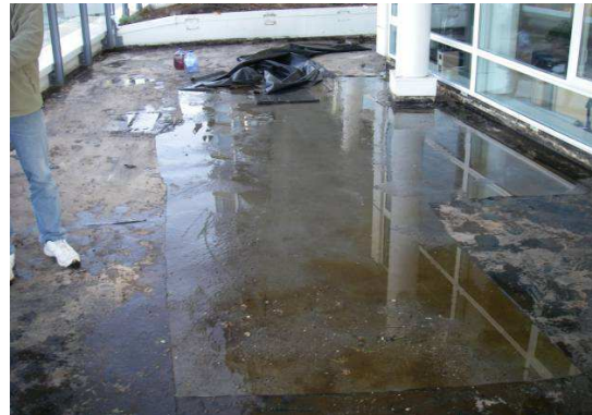
Figure 4: Water beneath blistered membrane
