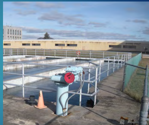
Flocculation Basin 35 MGD Flow Rate/Basin
