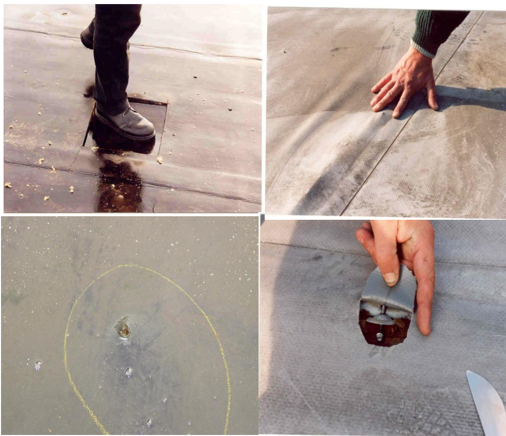
Figure 1: Roof failures in single-ply/mineral wool roofs showing insulation collapse due to frequent foot traffic and the screw heads penetrating the single-ply membrane (Source: Hendriks, 2010)
