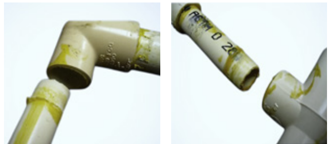
Images 22 and 23. Insufficient Cement/Dry Joint
