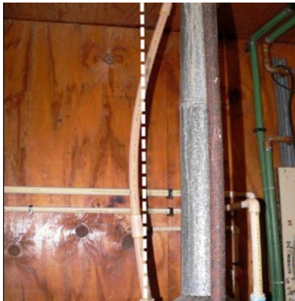
Image 12. Pipe Installed Near High Heat
