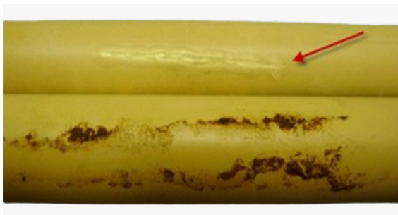
Image 2. Damage From Plasticizer Contact
