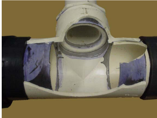
Figure 13: Dry Joint, no fusion of pipe and fitting.
