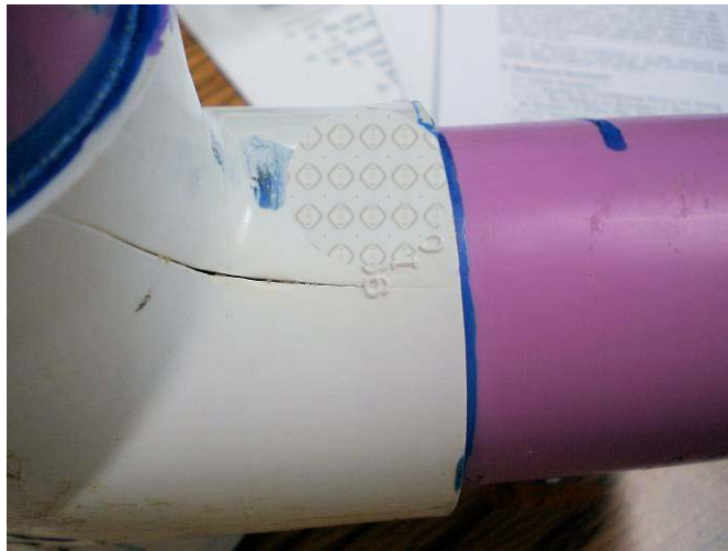
Figure 2: Classic long term failure
