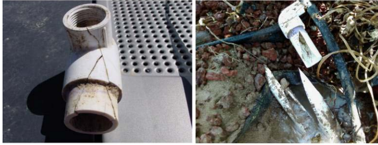
Figure 7: Breaks due to freezing water
