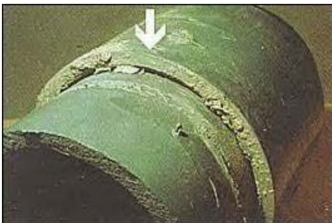
Figure 22: Insufficient Solvent cement was used.
