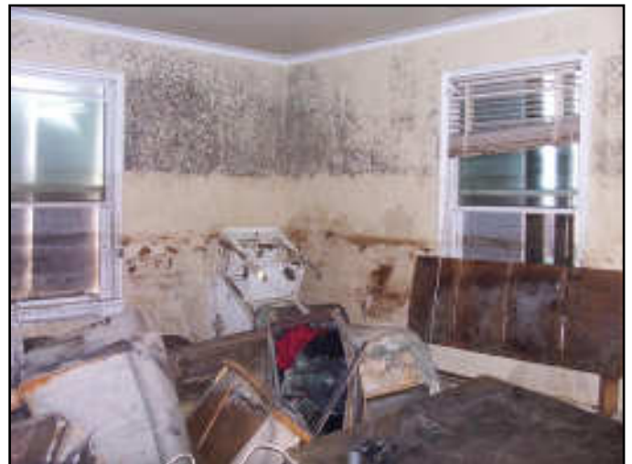
Figure 1. Typical flood damage to furniture and interior walls (Hurricane Katrina).
