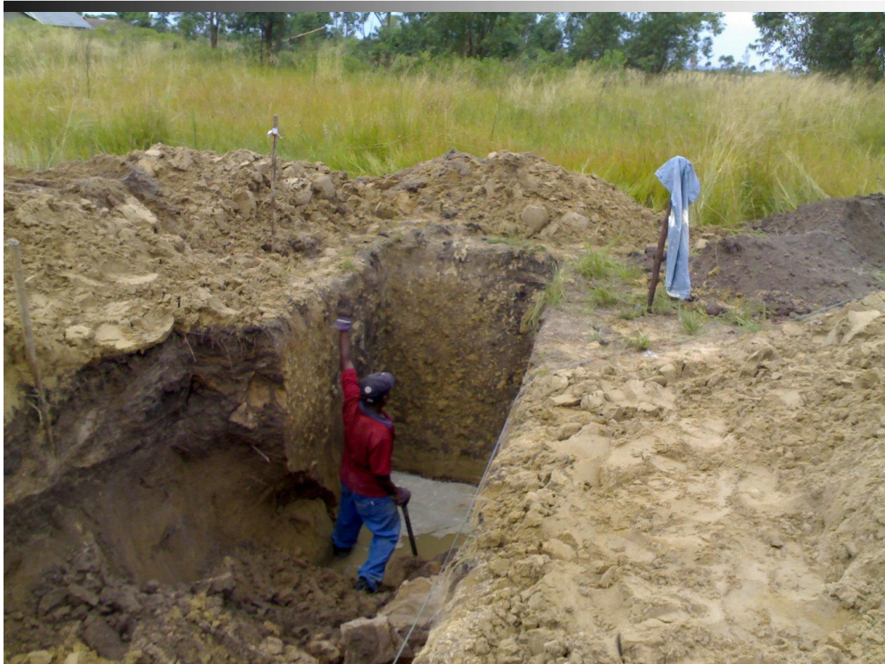
Trench collapse, Umhlathuze Municipal area, 2007 (Umhlathuze Municipality Excavation H&S Seminar Delegate, 2007)
