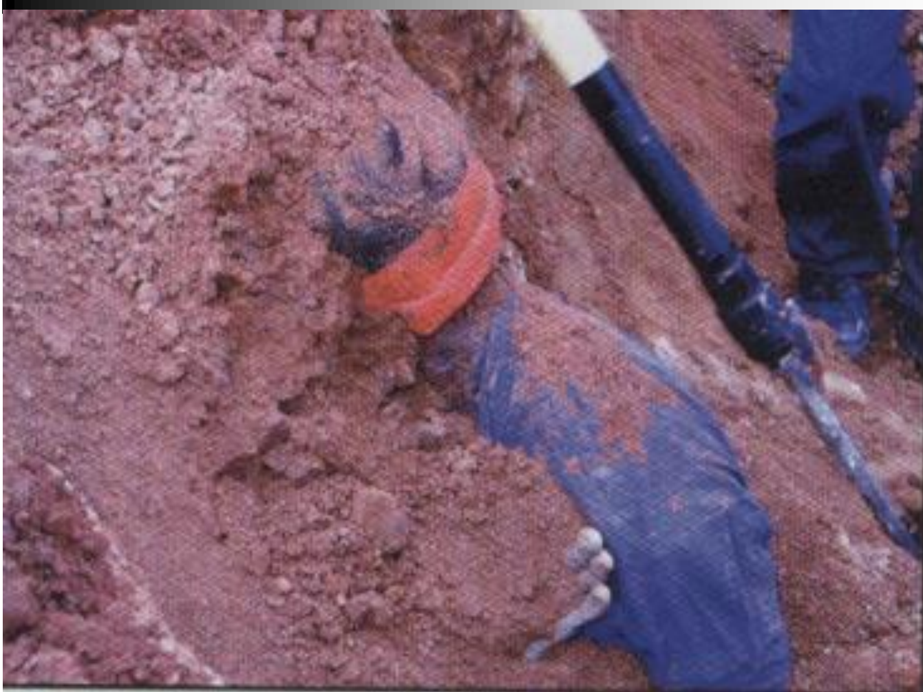
Trench collapse, Klein Brak River, March 2005 (Myer, 2005)
