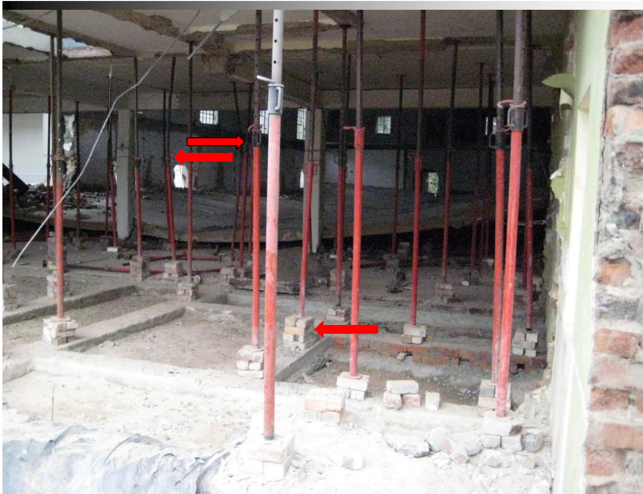
Stellenbosch Collapse (Anonymous, June 2008)
