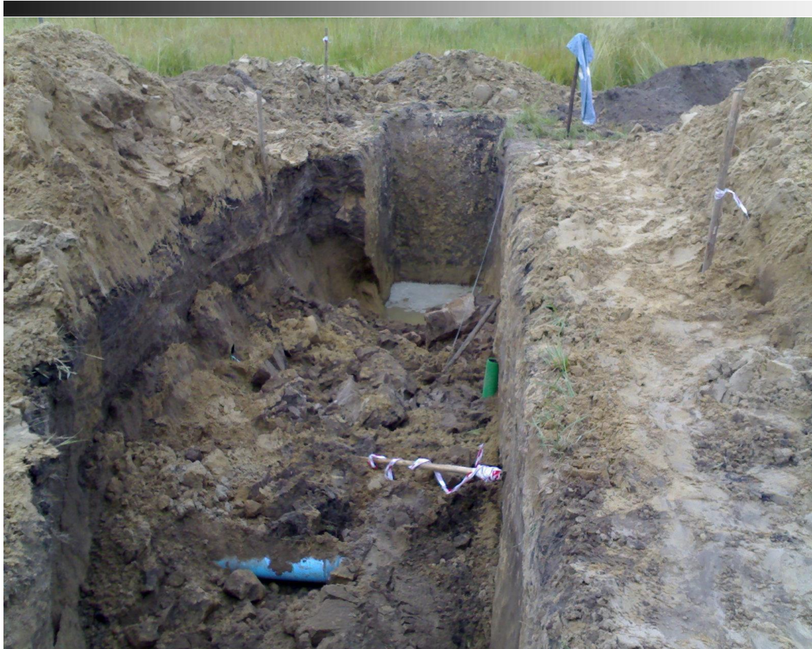
Trench collapse, Umhlathuze Municipal area, 2007 (Umhlathuze Municipality Excavation H&S Seminar Delegate, 2007)
