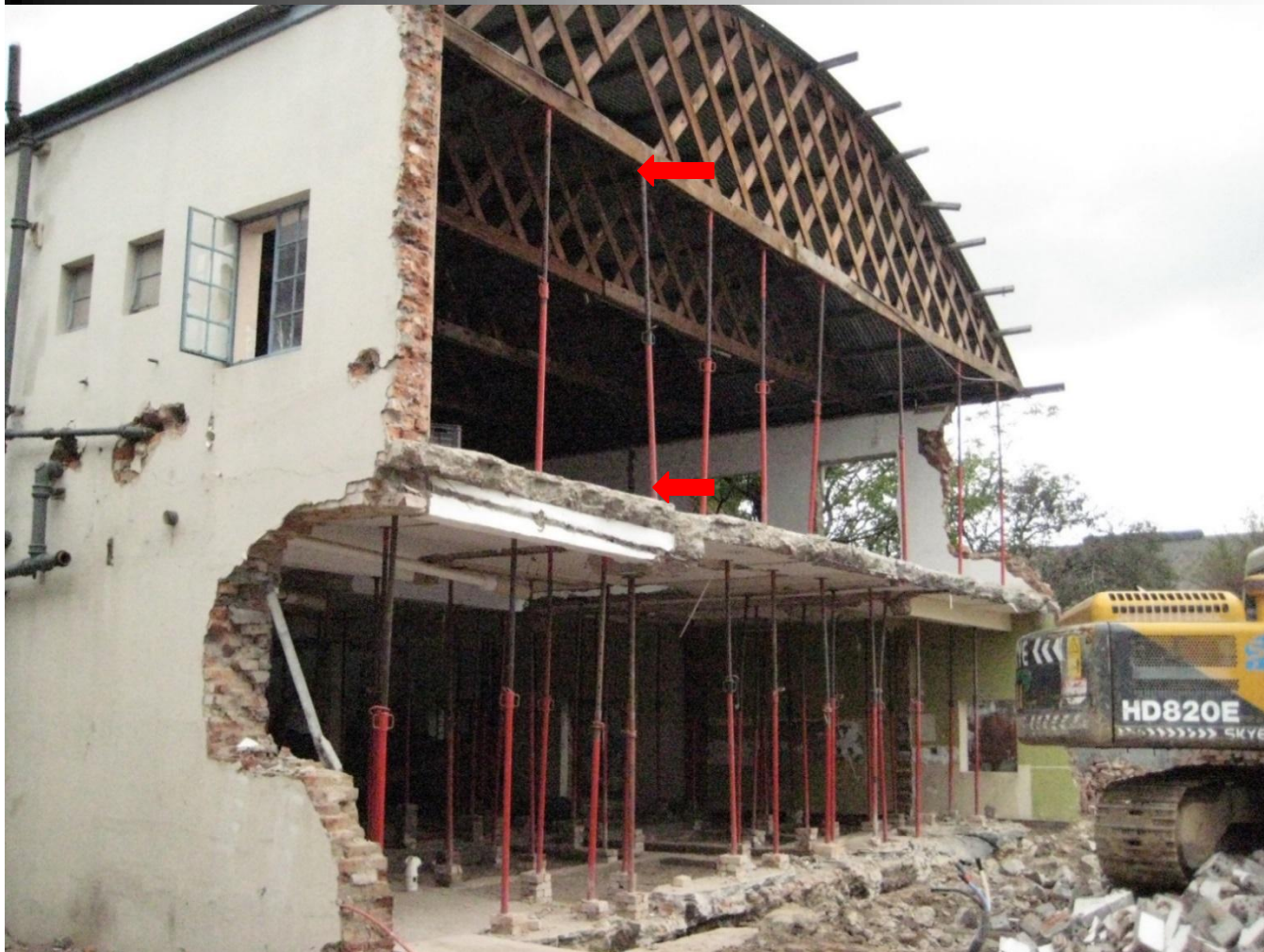
Stellenbosch Collapse (Anonymous, June 2008)
