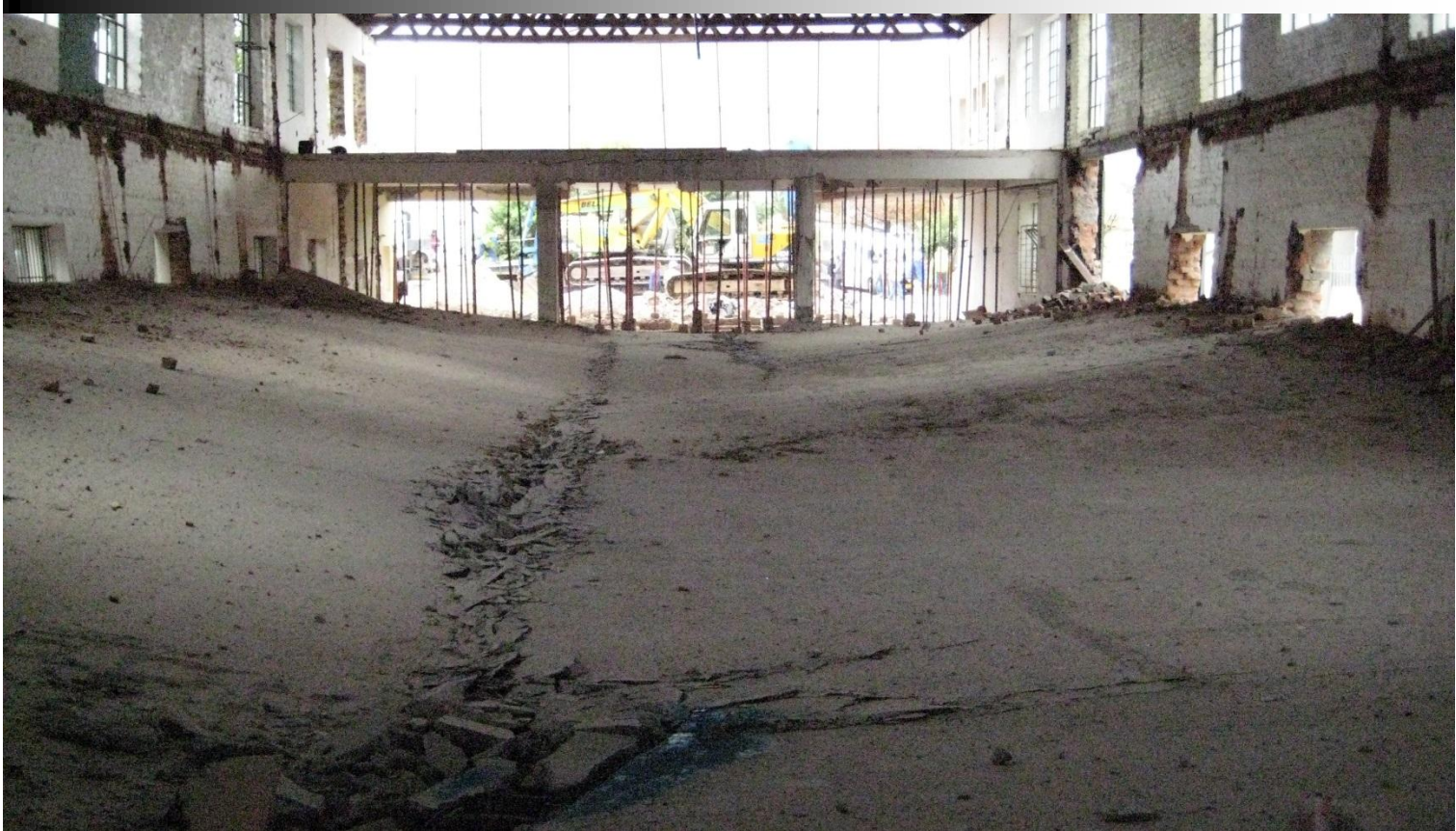
Stellenbosch Collapse (Anonymous, June 2008)
