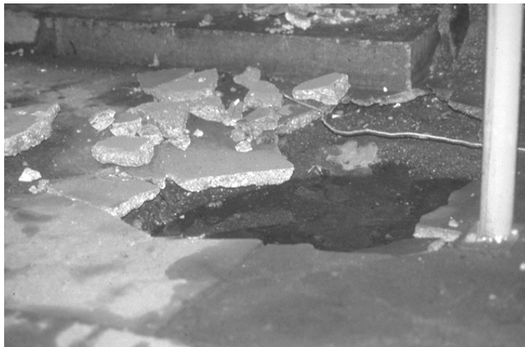
Figure 1-19. This basement floor broke from hydrostatic pressure
