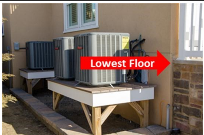
Heat pumps elevated, but lower than the lowest floor. Photo by Liz Roll/FEMA
