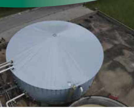
Clarifier & Tank Covers
